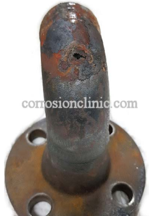
Figure 1a FAC at pipe elbow
